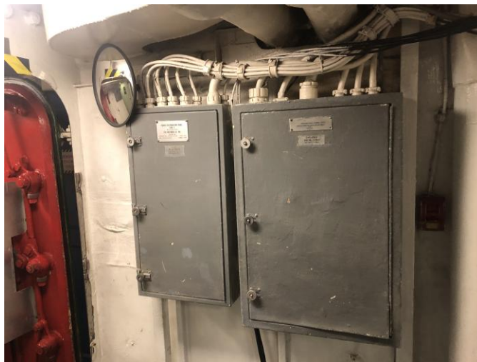
Figure 3: U.S.S. Midway (CV 41) Power Panel (Photo by Norbert Doerry)
