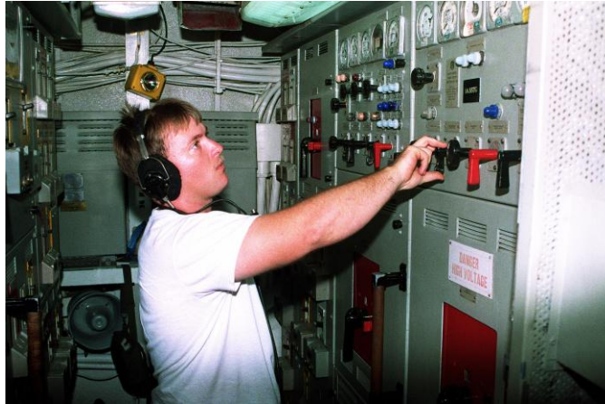
Figure 1: U.S.S. Goldsborough (DDG 20) Ship Service Switchboard (Image is in the public domain)
