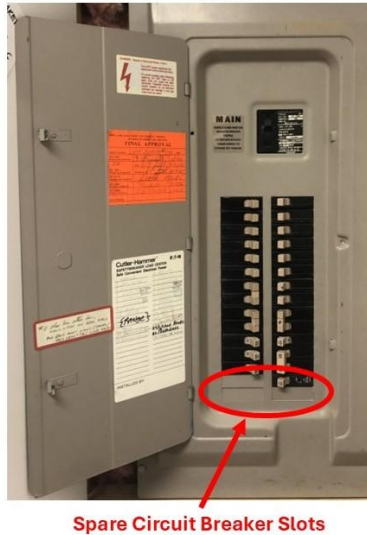
Figure 6: Spare slots for circuit breakers in a home power panel (Photo by Norbert Doerry)
